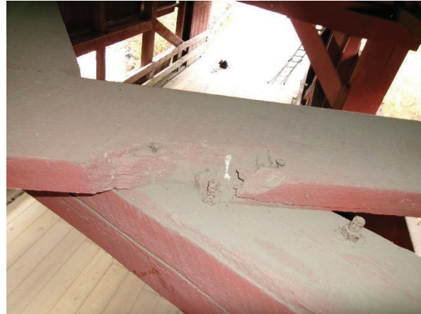
Broken Connection at Cross Beam and Diagonal
