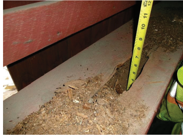
East Truss Top Chord Rot
