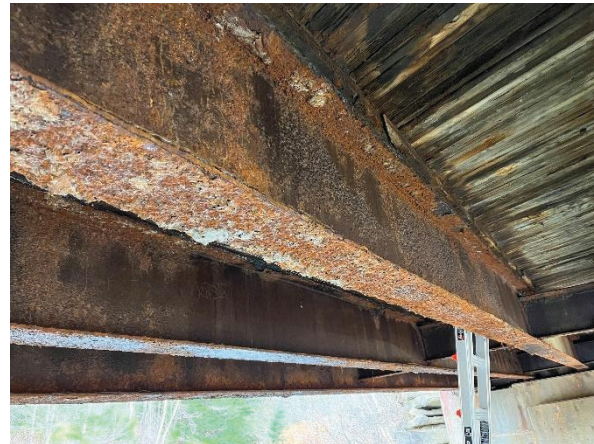
Interior Beam Rusting
