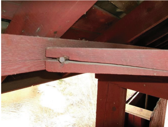
Split in Cross Beam
